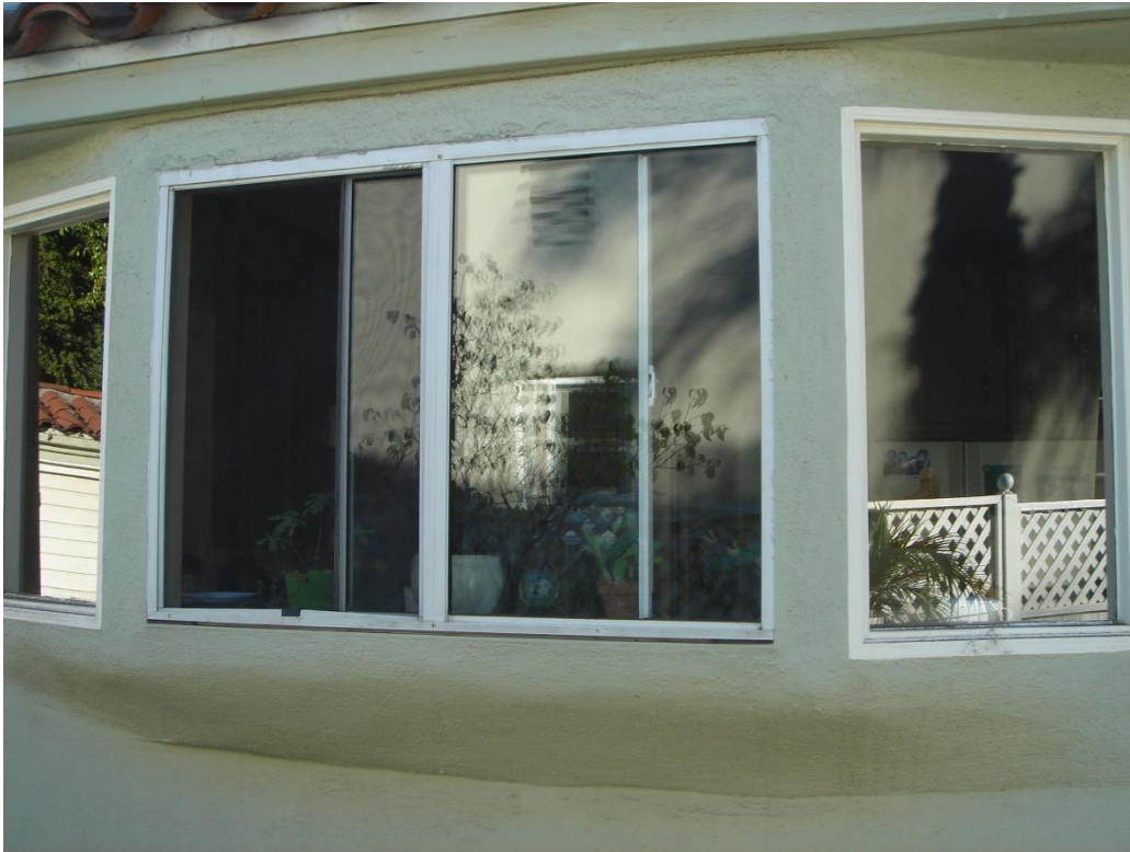
Existing Kitchen Window. Fixed Single Pane Side Windows. Center Aluminum Sliding Window.
